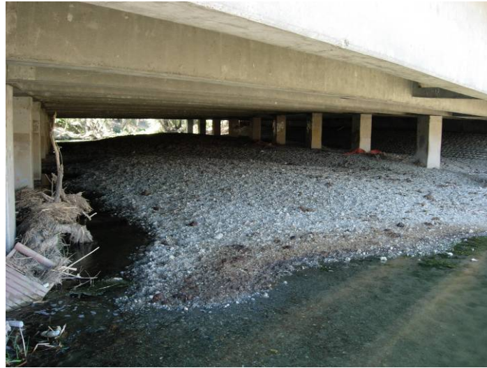
Figure 3-15: Sediment Deposits along Arroyo las Positas at the I-580 Crossing
