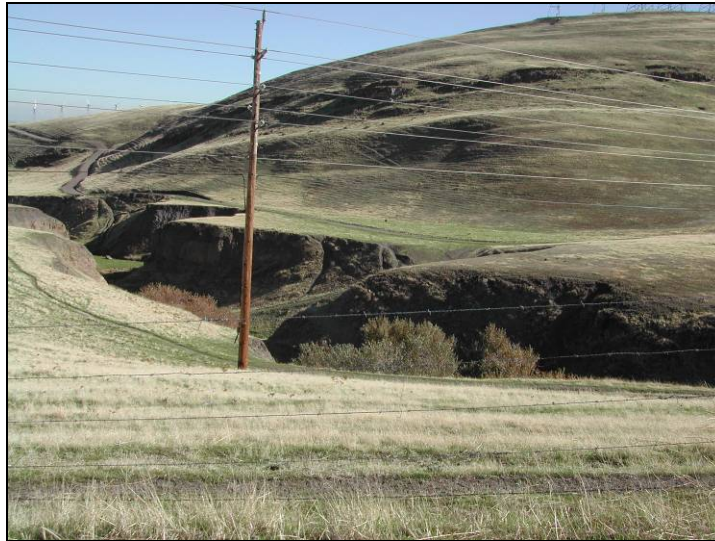
Figure 3-19: Bank Erosion in Patterson Run (Line Y-1)
