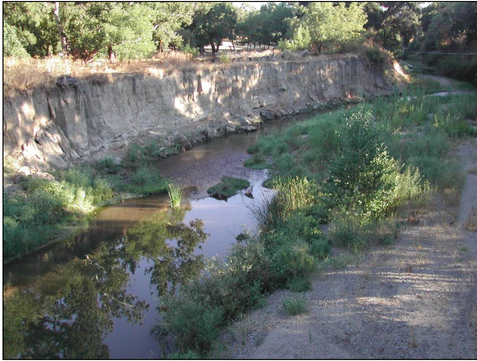
Figure 1-7: Bank Erosion along ADLL Downstream of Bernal Bridge
