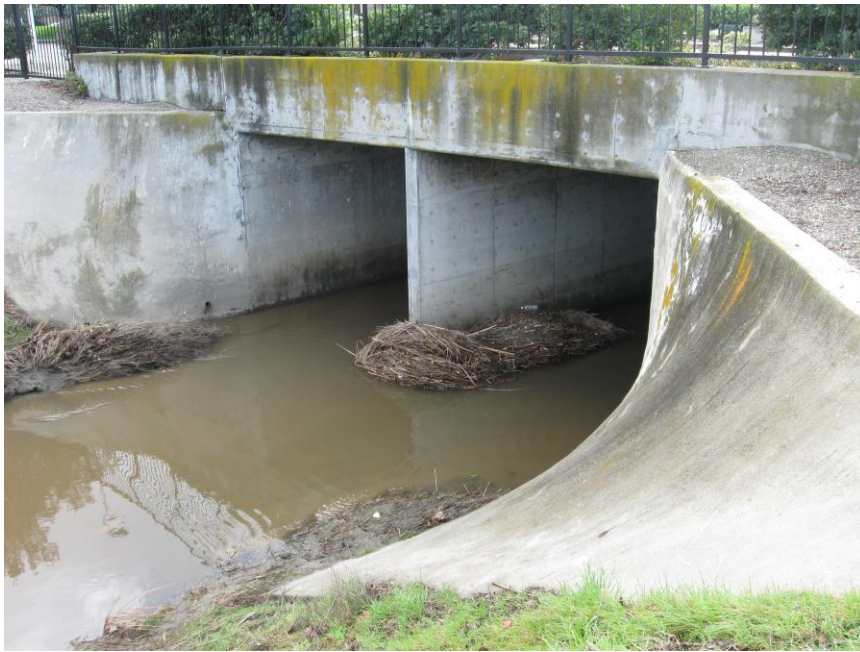
Grasses and weeds block a channel pier and prohibit flow in Chabot Canal in Pleasanton after a typical small rain storm
