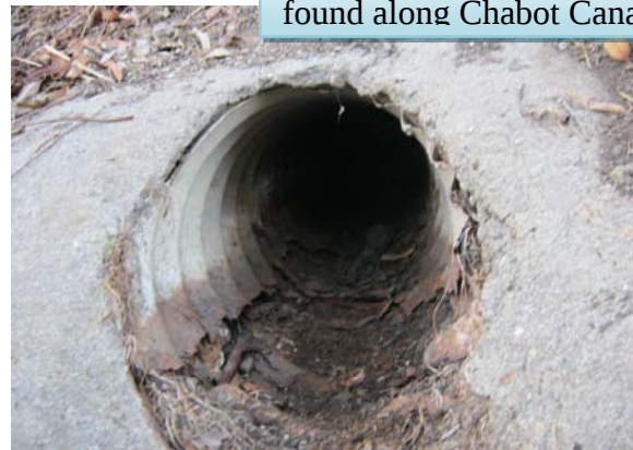
Corroded storm drain pipe found along Chabot Canal
