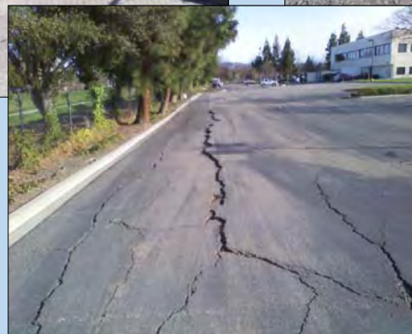
DISTRESS EXAMPLES – Concentrations Near Large Exposed Unpaved Areas, Slopes (e.g. Canal Banks) In Areas With Expansive Soils, +/- Tree Rows
