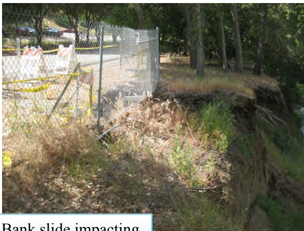
Bank slide impacting Foothill Road
