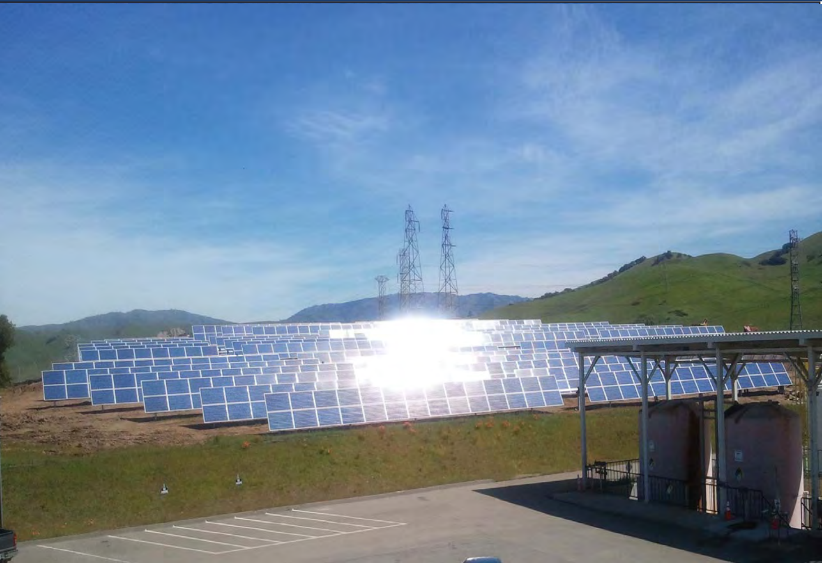
New Solar Panels at the Del Valle Water Treatment Plant
